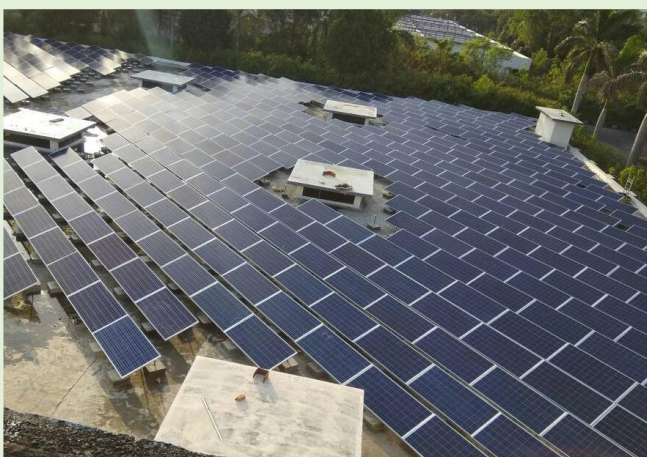
Solar Panels at Katagram Water Works
