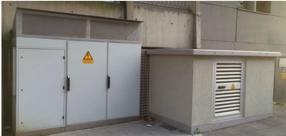
Fig. 12 Charging station (Heliox charging station at Cologne – Germany)
